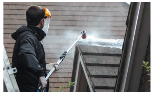
These growths on a roof can result in costly repairs
